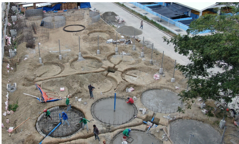
Aerial view of the ongoing construction of the new shrimp broodstock facilities in SEAFDEC/AQD. Photo by JF Aldon
