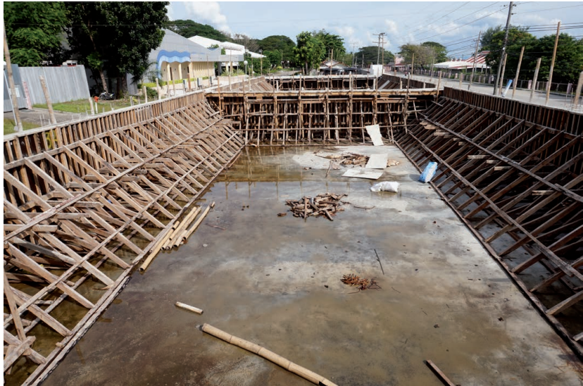
Construction of new milkfish broodstock tanks at the Tigbauan Main Station as of December 2020. Four new units of 500-ton broodstock tanks will host at least 320 new milkfish breeders to beef up SEAFDEC/AQD's capacity to produce eggs and larvae.
