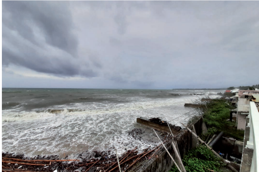
Climate change impacts may include sea level rise which, when compounded with more severe weather events, could severely affect coastal aquaculture facilities. Shown here is a storm surge threatening the seawall of the Tigbauan Main Station of SEAFDEC/AQD.
