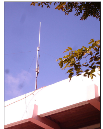
WiFi antenna at the dormitory rooftop
