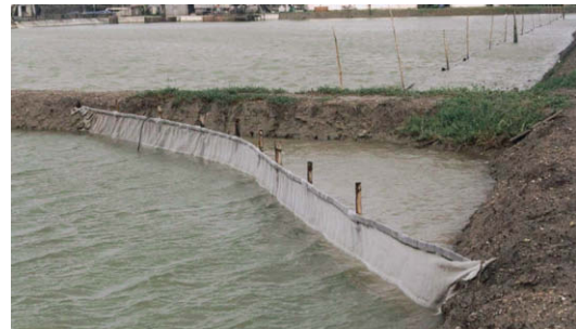
Corner Sludge Collector
