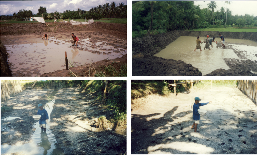
Figure 4. (Clockwise from top left): Pond draining and levelling, repair of gates and dikes, eradication of pests, and liming
