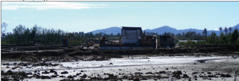
Climate change is upon us: damage to the dikes in an experimental pond in Iloilo, Philippines caused by super typhoon Yolanda / Hainan in late 2013
