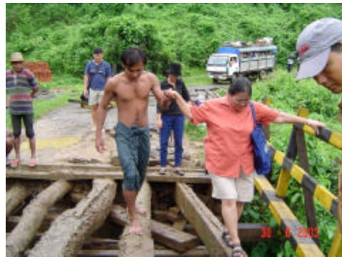
Crossing the broken bridge on the way to Toungguk was a reminiscent of the Tigbauan Bridge incident
